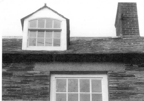
'Pitched' dormers are the most typical in the area but are more complicated to construct. Note the small size of the dormer compared to the window on the main facade. Lead or slate are suitable materials for the dormer cheeks.
