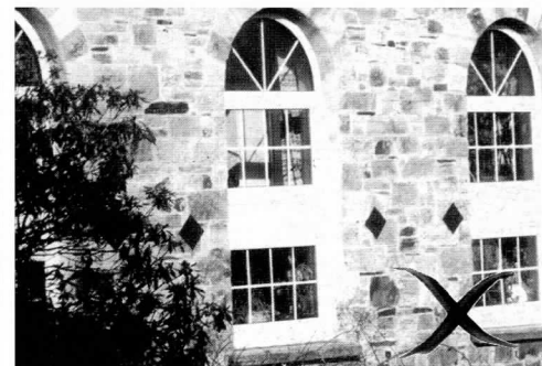
Avoid incorrectly detailed fan-headed windows.
