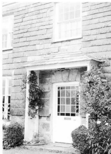
A Victorian door partly glazed with etched stained and cut glass panels. Retain these elements if at all possible.
