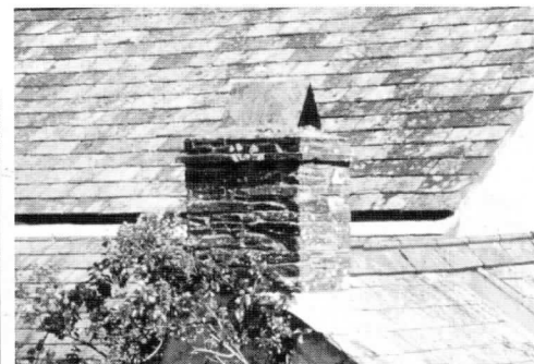
A simple stone stack with a pair of tilted slates to keep the worst of the rain out - a traditional detail.
