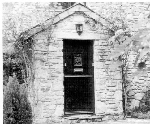
A modern porch built in the vernacular style using slate verges and granite lintol.
