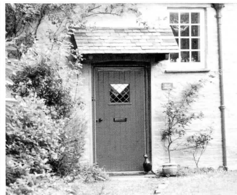
A simple lean-to slate canopy with timber bracket supports on a traditional cottage. Note that gutters are not required on very small areas of roof, helping to create a lighter uncluttered appearance.
