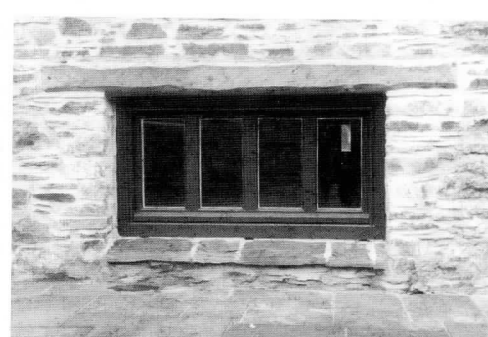
Unpainted adzed timber lintel and slate cill details on a barn conversion.
