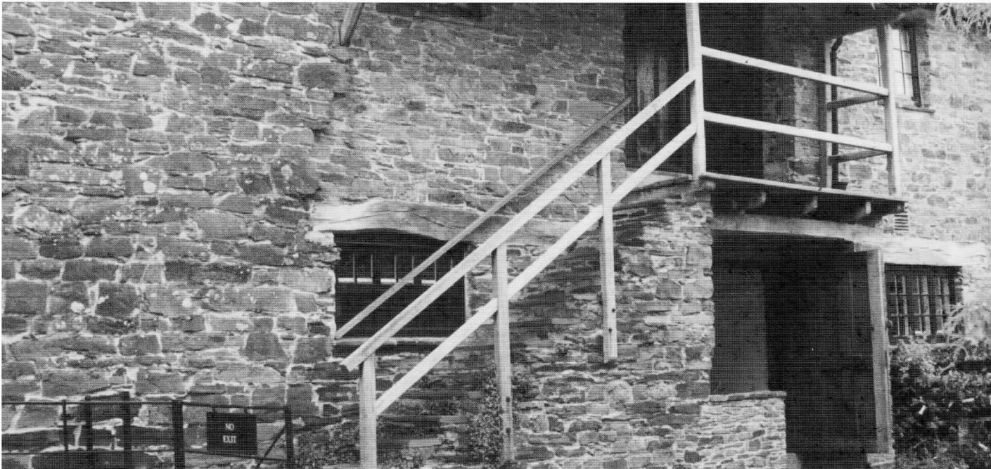
Coursed rubble walling of local stone at Cotebele. Note the substantial oak lintels to the door and window openings.
