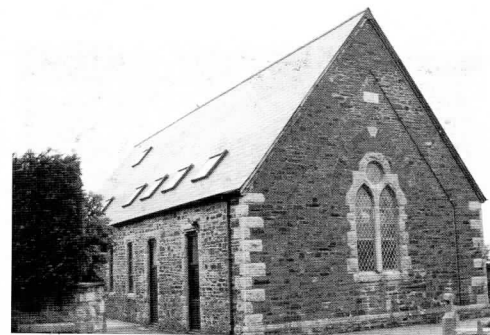
The 'reordering' of this large chapel at Upton Cross has included the insertion of an additional floor to create rooms in the roof, while retaining the original fabric and character.
