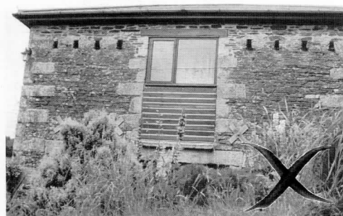
Avoid the use of horizontal tongue and groove boarding and decorative lead flashings on conversions - they are too domestic.
