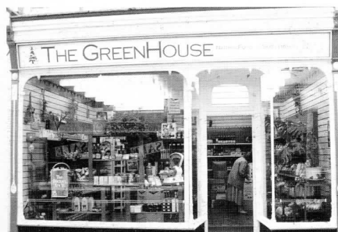
The cast iron detail on this Victorian shop front and the mosaic tiled door step are full of character, and add to the overall streetscape.
