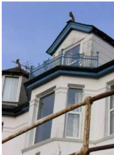
21: Cast iron work on bay windows – Art Nouveau style in this case
