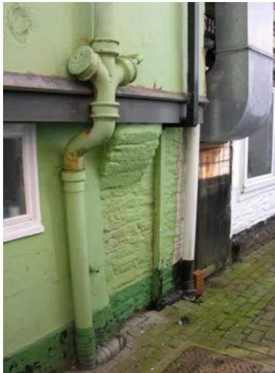
23: One of the town's oldest buildings is disfigured by clutter
