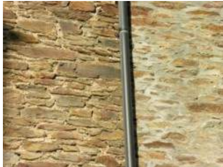
25: Bad cement pointing is ugly and harmful
